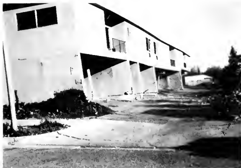
Photo 15. Severely damaged and leaning modern apartment building, now razed, formerly at southeast corner of Foothill Boulevard and Harding Avenue (locality 81). View northeast. Fault break of Sylmar segment extended through corner of building in for carport and crossed Harding Street to right of camera point. Building was constructed on older alluvium.
